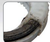
Broken bearing Defektes Lager Viottunut laakeri
